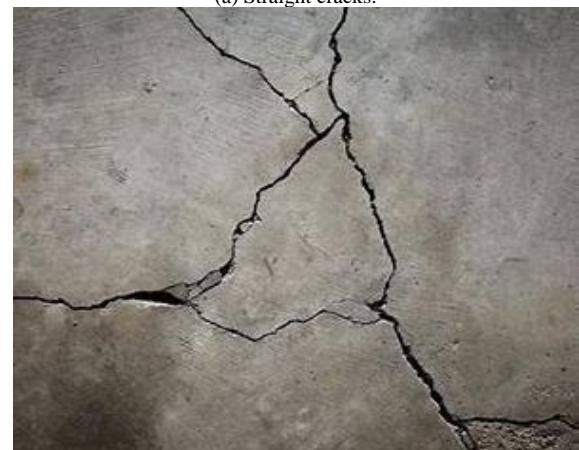
(b) Reticulated cracks.
