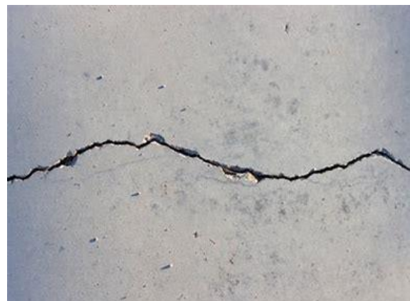
(a) Straight cracks.
