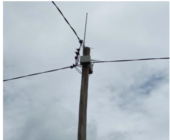
Fig. 4. LoRa Base Station Installed at the Pole.
