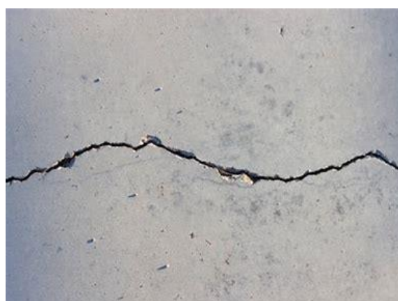
(a) Straight cracks.
