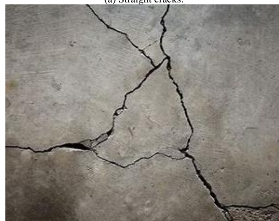
(b) Reticulated cracks.
