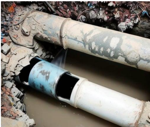
Fig. 2. Water pipe crack.
