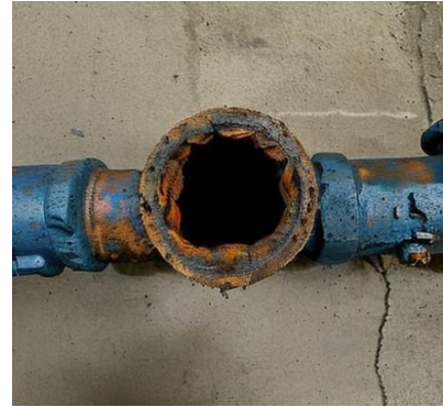
Fig. 3. Water pipe corrosion.
