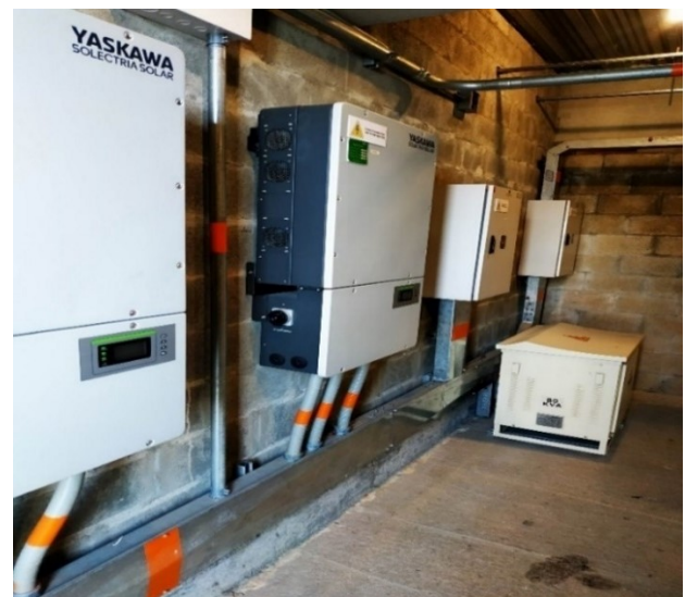
Fig. 2. Three-phase solar inverters and grid-connected electrical system.
