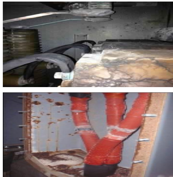
Fig. 2. Apparition of the dew inside the electric cells
