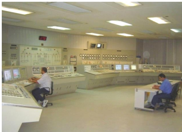
Fig. 3. Control room of the TPP
